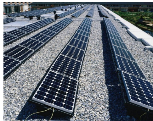
Azienda 200 kWp (BS)
