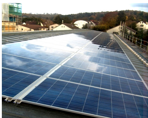
Azienda 20 kWp (BS)
