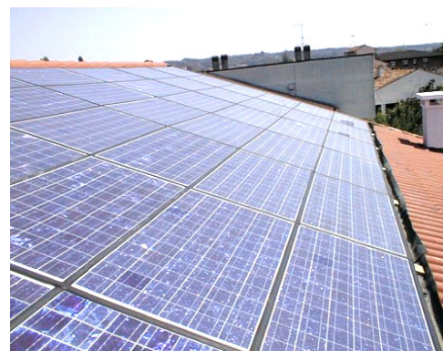
Azienda 34 kWp (BS)
